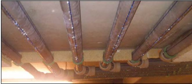
Illustration 6.5 Condensation on cold water lines
