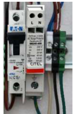
Figure 50. AC Wiring to Terminal Blocks
