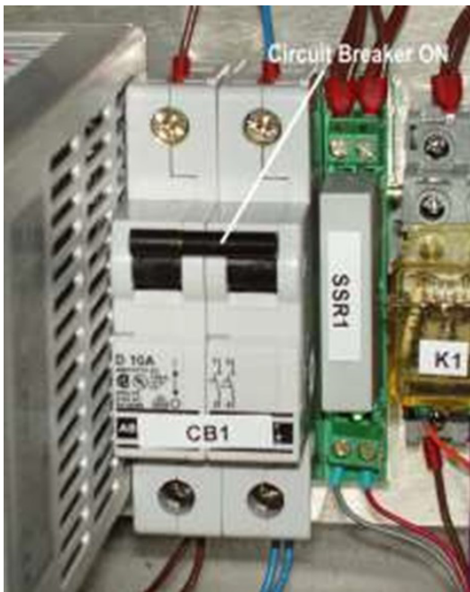
Figure 9. Circuit Breaker in ON Position
