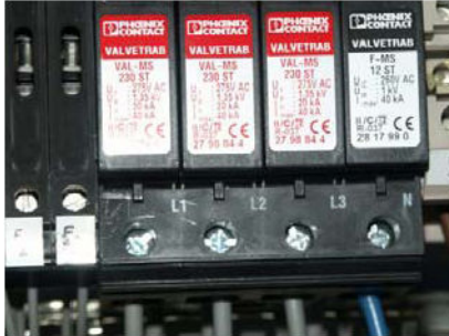
Figure 48: Over-voltage protection cartridges
