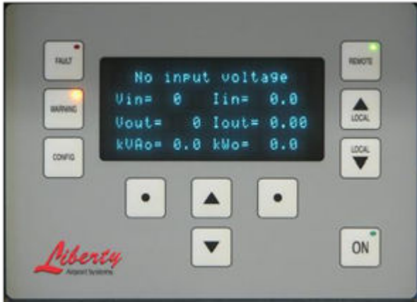
Figure 18: Typical Warning Message - No Input Voltage
