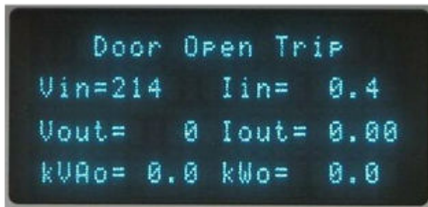
Figure 12: Display showing Door Open Trip
