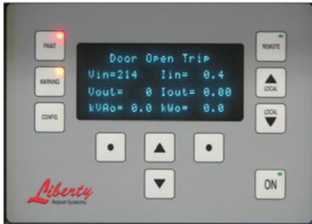
Figure 19: Typical Fault Message - Door Open Trip
