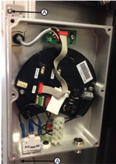
Figure 36: Electronic Box in Sign Frame
