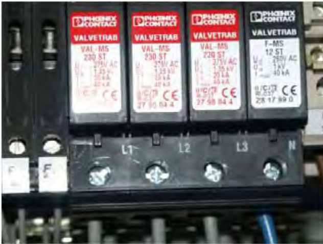
Figure 50: Over-voltage protection cartridges
