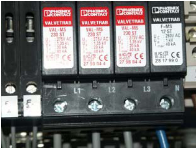
Figure 50: Over-voltage protection cartridges
