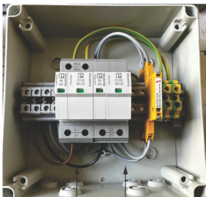
Figure 10: OLP Unit Surge Protection Devices
