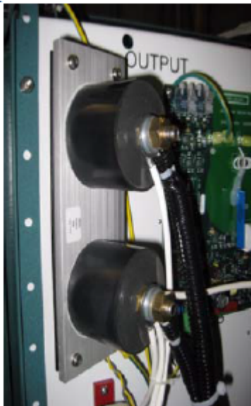
Figure 32: Output Lightning Arrestors
