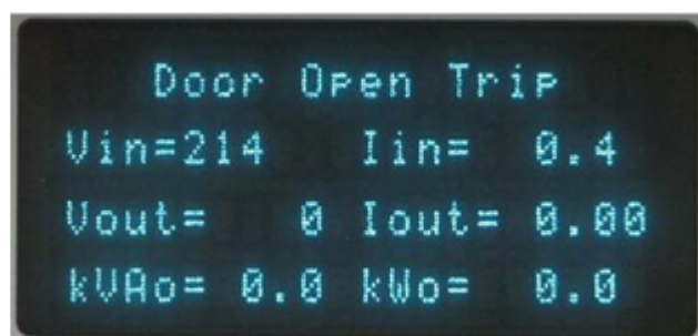
Figure 12: Display showing Door Open Trip
