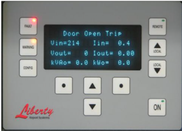
Figure 20: Typical Fault Message - Door Open Trip
