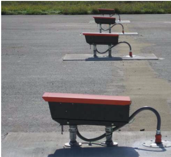
Figure 12: Example PAPI Installation
