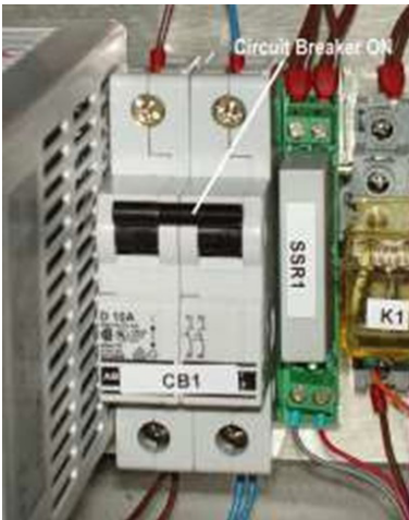
Figure 11. Circuit Breaker in ON Position
