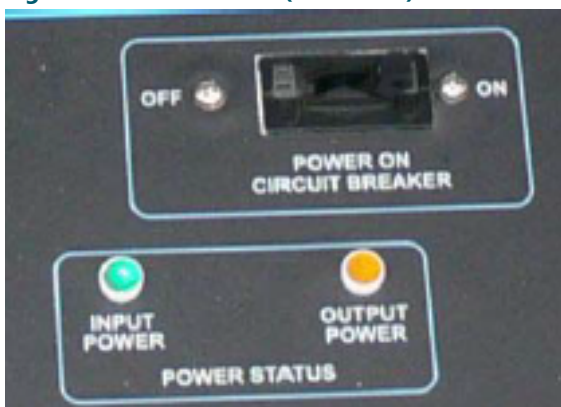
Figure 3: Circuit Breaker (Power ON) switch and Power Indicators
