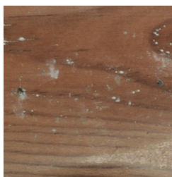
Surface mould/Moho superficial/ Moississures superficielles/ Oberflächlicher Moder/Muf fa su- perficiale/Oppervlakte-schimmel/ Bolor superficial
