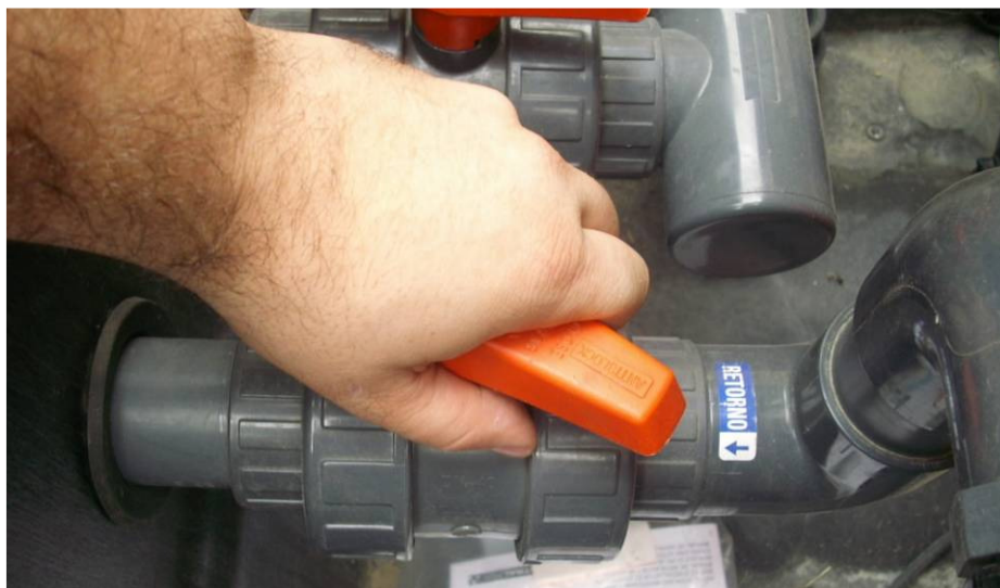
Fig. 23.- Close the return to pool valve.
