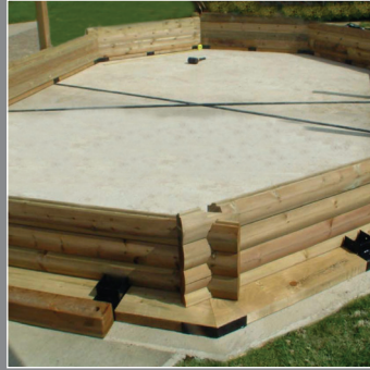
Lay out the base structure and start to build the wooden sections which fit together perfectly
