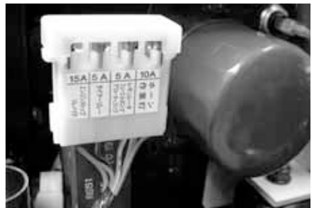
Isn't the fuse blown? (Photo 4)
