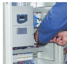
CONTROL PANEL WITH FREQUENCY IN INVERTER
