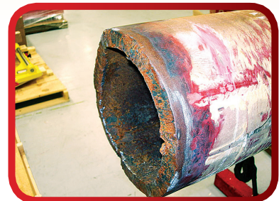
Hot torch cutting requires grinding and produces an undesirable heat affected zone.
