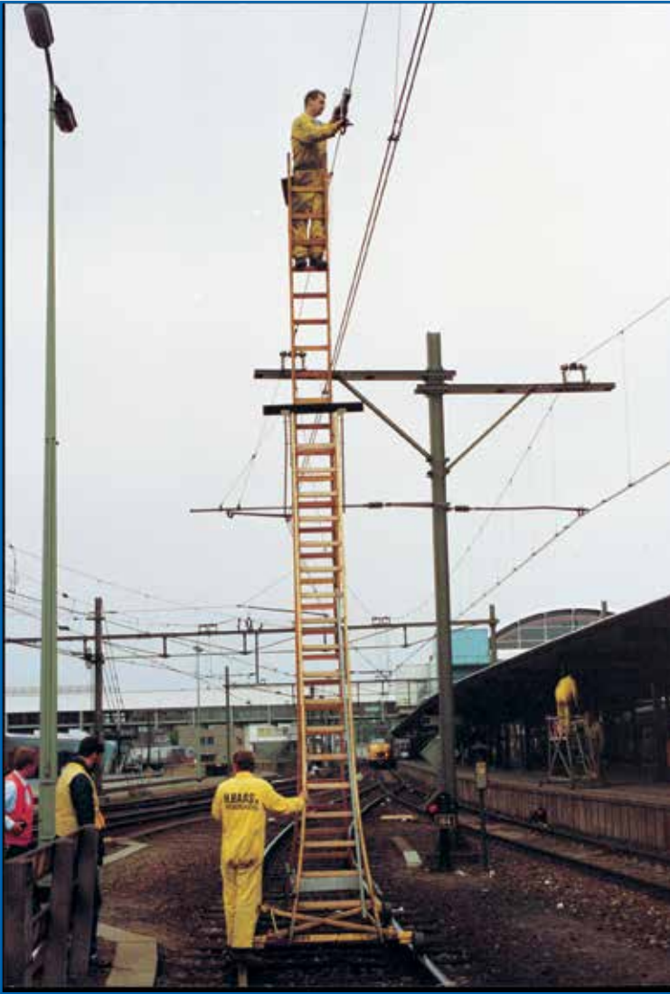
The PIAB RTM 20D is in use when installing/inspecting suspension and catenary ropes.
