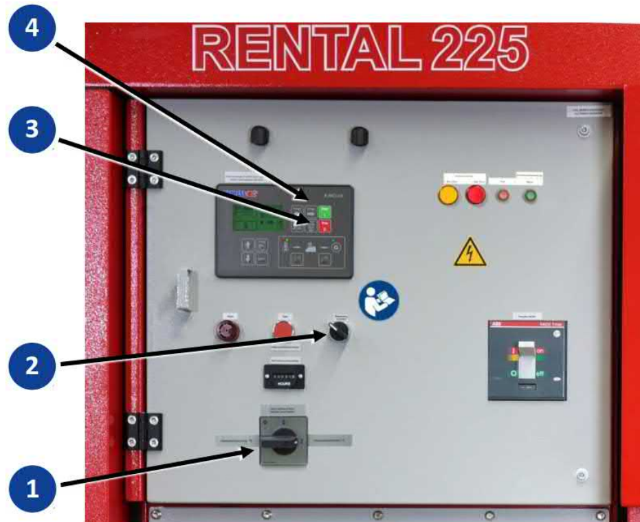
Fig. 7-2 Manually starting and stopping the power generator
