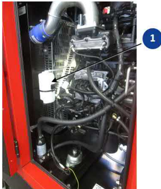
Fig. 10-3 Checking the coolant
