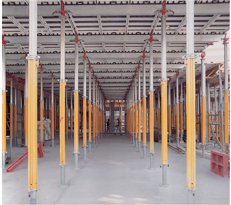
MULTIPROP 350 with Base MP 50 together with SKYDECK being used to shutter a slab with a clear height of 4.10 m.
