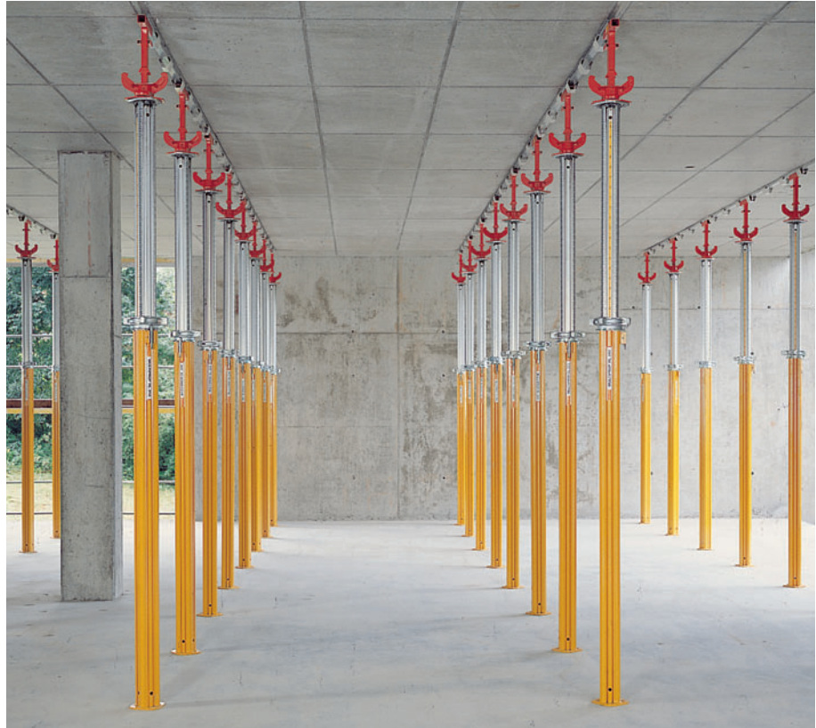
MULTIPROP 350 and SKYDECK slab formwork after striking. Only 0.29 props/m 2 for slabs up to 40 cm deep.
