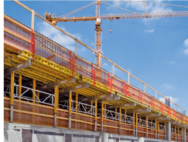
MULTIPROP towers with MPB Aluminium Beam as main beam and GT 24 as cross beam.
