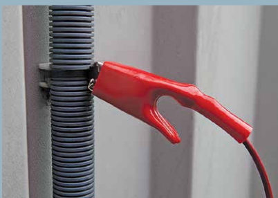
Small diameter cable tracing techniques
