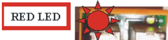
Relay Inside Ground Control Box
