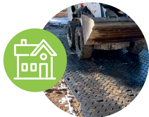
Residential Contracting Water, Gas, Electricity, Powerline, Landscaping
